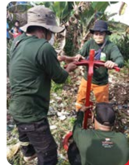
Training for trainers to build The Akhlag well in Pelalawan, Riau. It is the source of water during fire but also an effective way to create water stocks in peatlands and retain soil moisture on dry seasons
